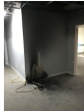
Area where heater had been situated.
