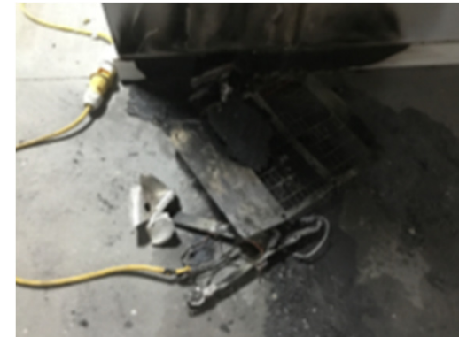
Remains of the heater
